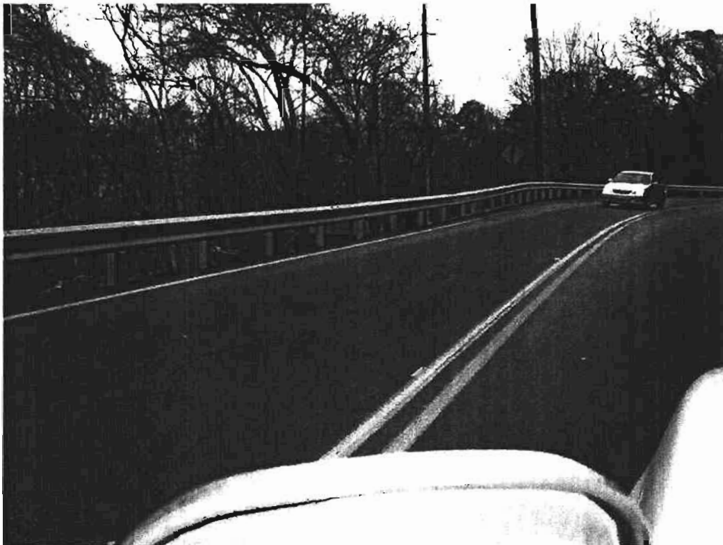
Figure 2. View of new sliding along State Route 8 in the area of the “Space House Slide”
